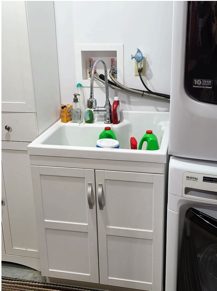
Figure 31 Laundry sink. (Skilled Trades BC, 2021) Used with permission.
