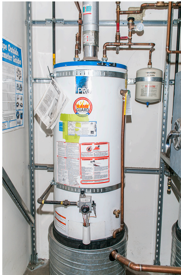
Figure 9 Hot water tank installation with potable expansion tank and seismic restraint kit. (Skilled Trades BC, 2021) Used with permission.
