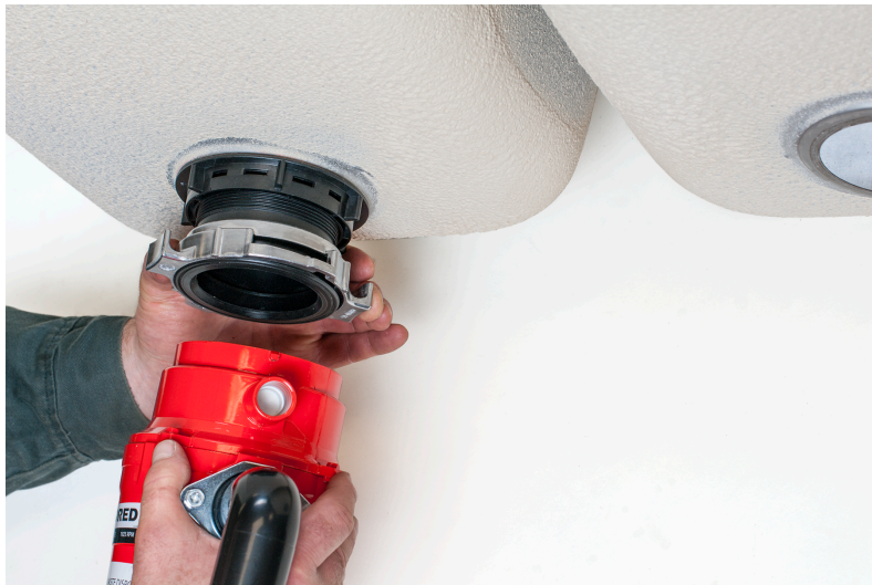
Figure 4 Mounting the garburator to the outlet fitting. (Skilled Trades BC, 2021) Used with permission.
