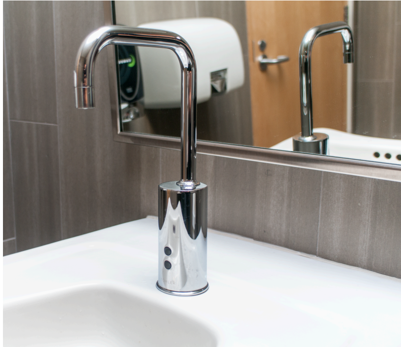
Figure 70 Sensor-activated faucet. (Skilled Trades BC, 2021) Used with permission.
