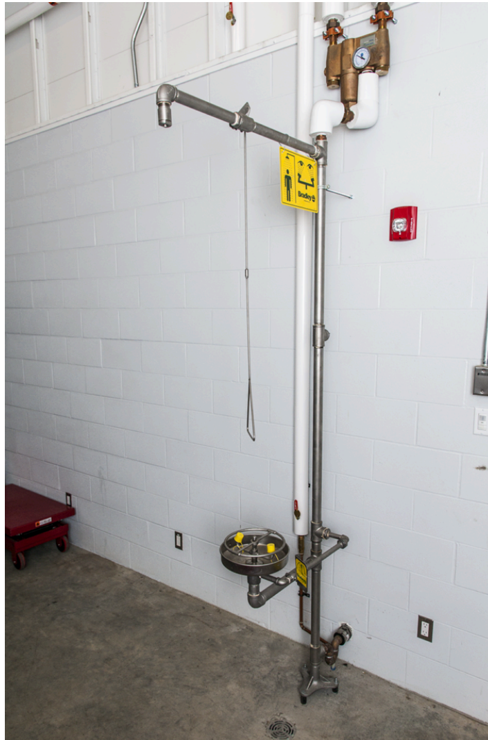
Figure 48 Emergency shower and eyewash station. (Skilled Trades BC, 2021) Used with permission.
