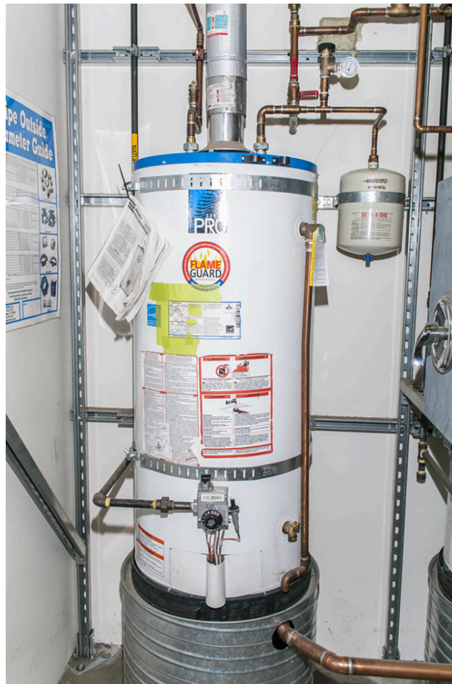
Figure 9 Hot water tank installation with potable expansion tank and seismic restraint kit. (Skilled Trades BC, 2021) Used with permission.
